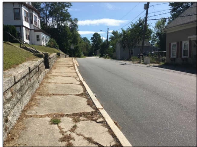
Poor sidewalk conditions are found on most sidewalks in Millville, including Lincoln Street
